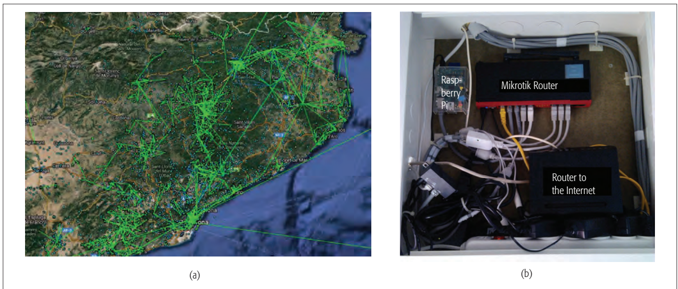
Figure 4. (a) Structure of Guifi.net around Barcelona (Spain); (b) junction box of a guifi.net supernode (Spain), including a Mikrotik wireless router, a Raspberry Pi used as proxy, and the router of the operator connecting to the Internet.
